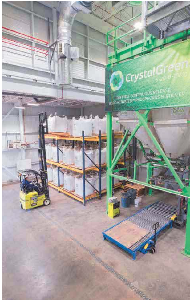
Minimal volumes of Crystal Green produced at the wastewater plant are stored before shipment
