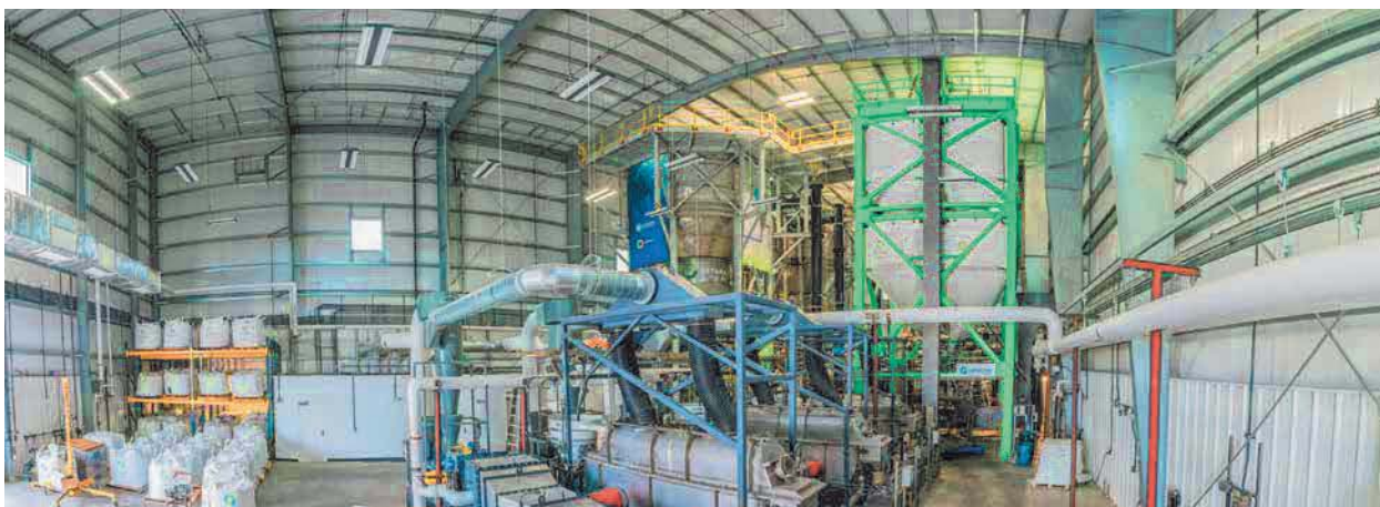
Ostara's Pearl technology transforms nutrient-rich wastewater from an Edmonton wastewater treatment plant into sustainable fertilizer. Photo courtesy of Black & Veatch
