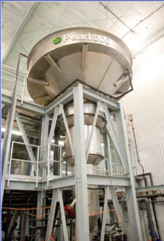
Three reactors installed in the facility have the ability to recover 1.5 tons of fertilizer on a daily basis.
