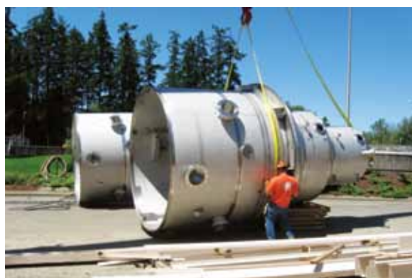
To maximize the production of fertilizer, CWS created the WASSTRIP process, which doubles the amount of phosphorous sent to nutrient recovery.
